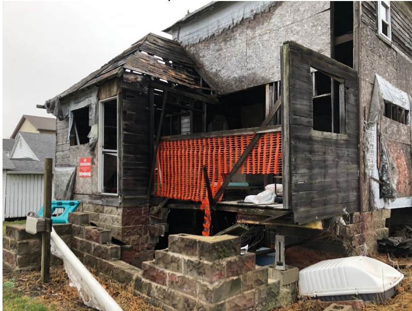
Outside view of structure. Foundation held up by jacks.
