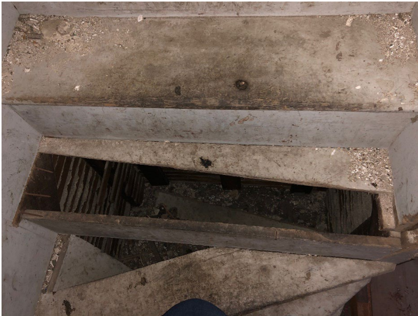
View of hole in the staircase.
