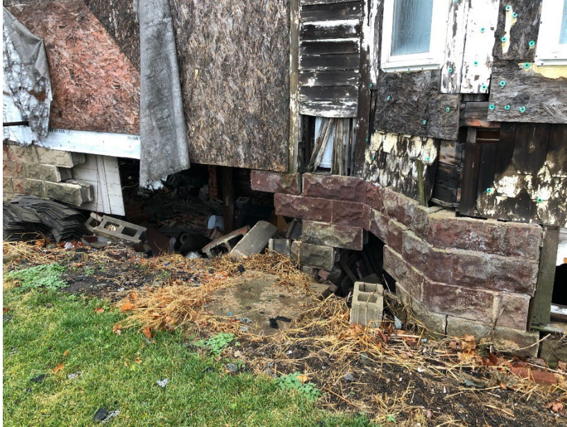
Outside view of missing foundation.
