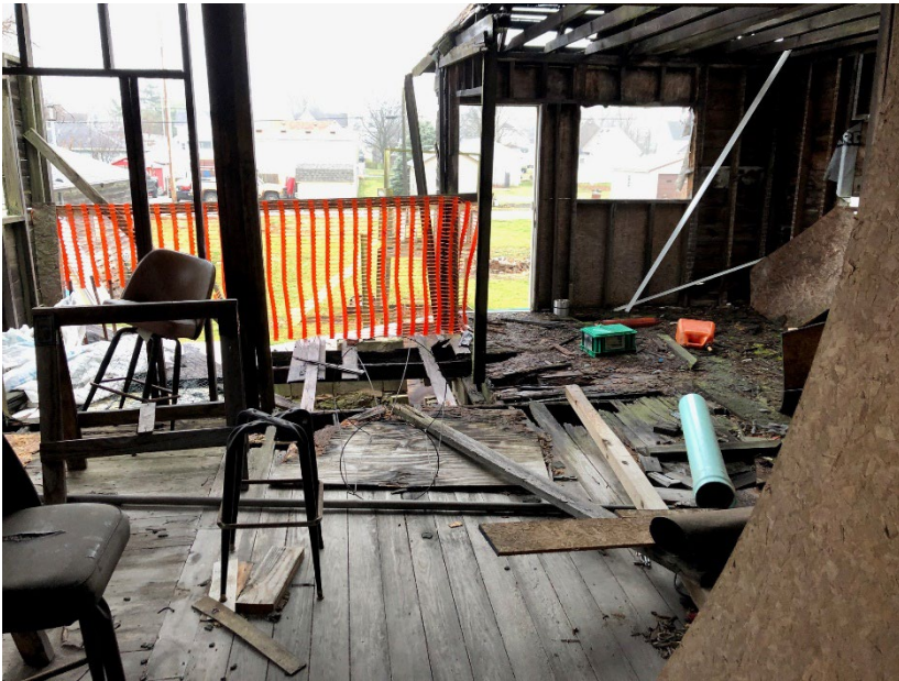
Interior of structurally unsafe residence.
